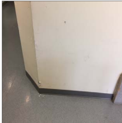
Photo 5 – Damaged asbestos-containing drywall joint compound and debris, Level 1 Easy Street Area, East Wing.
