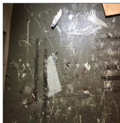
Photo 2 - Presumed asbestos-containing 12"x12" grey and dark grey flakes vinyl floor tile within Level 1 Room S105C.
