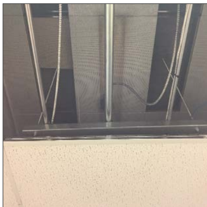
Asbestos-containing paper above metal pan ceiling tiles, First Floor Corridor.
