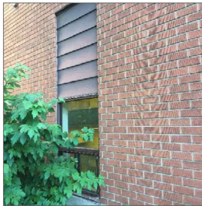
Asbestos-containing caulking at exterior window frame, Boiler House.
