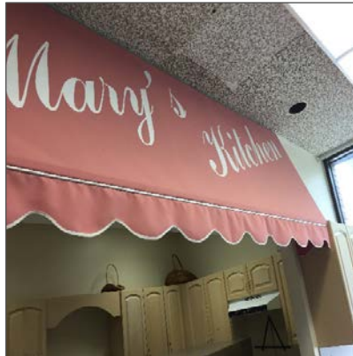
Non-asbestos 12" x 24" glued-on ceiling tiles with large fissure pattern, adhered with presumed asbestos-containing mastic, Level 1 Easy Street Area.
