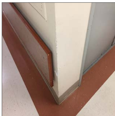
Photo 3 – Damaged asbestos-containing drywall joint compound on wall, Level 3 Corridor at Tub/Shower Room, West Wing.
