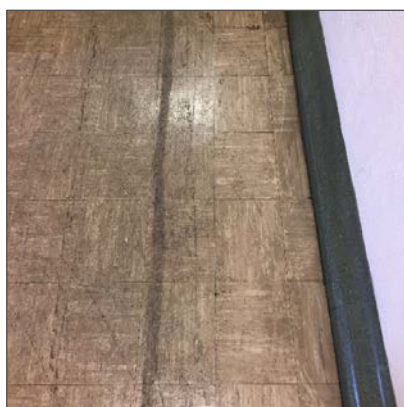
Photo 1 - Asbestos-containing 12"x12" white and beige streaks vinyl floor tile within Level 1 Corridor.
