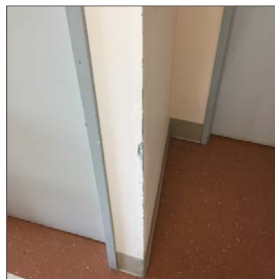
Photo 4 – Damaged asbestos-containing drywall joint compound on wall, Level 4 Corridor at Room E423, East Wing.
